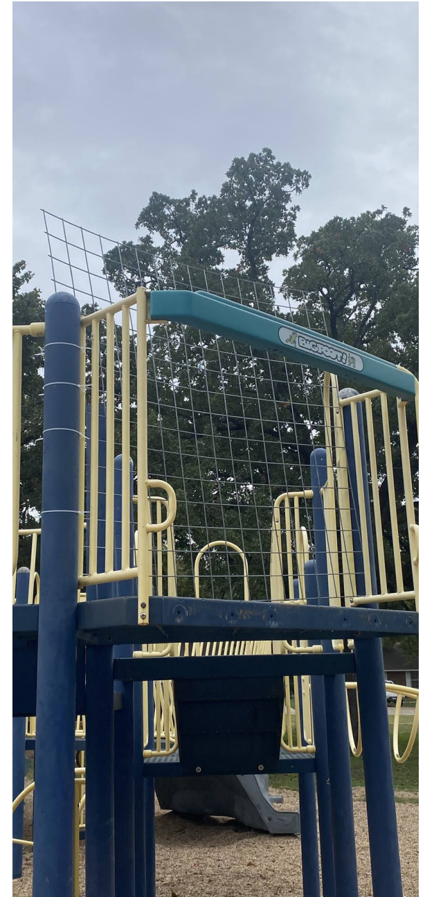
Needed maintenance at Veterans Park
