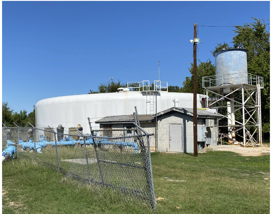
Rockdale Water Treatment Facility
